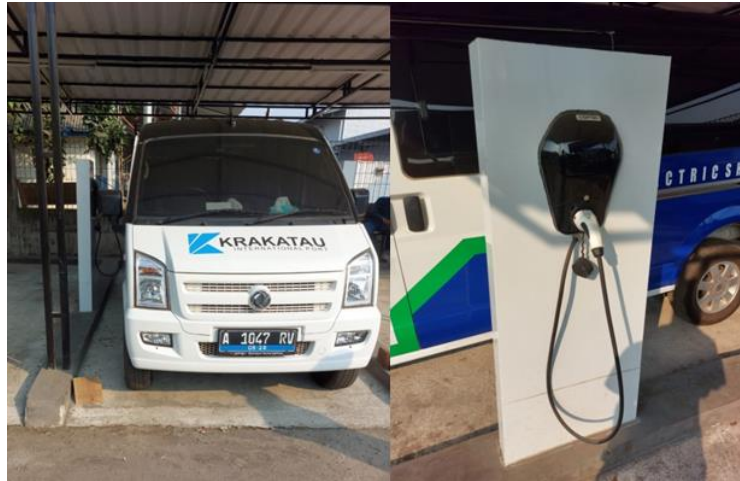
Electric Vehicle & Charging Station
