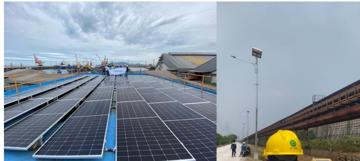
Solar Panels and Solar Street Lights
